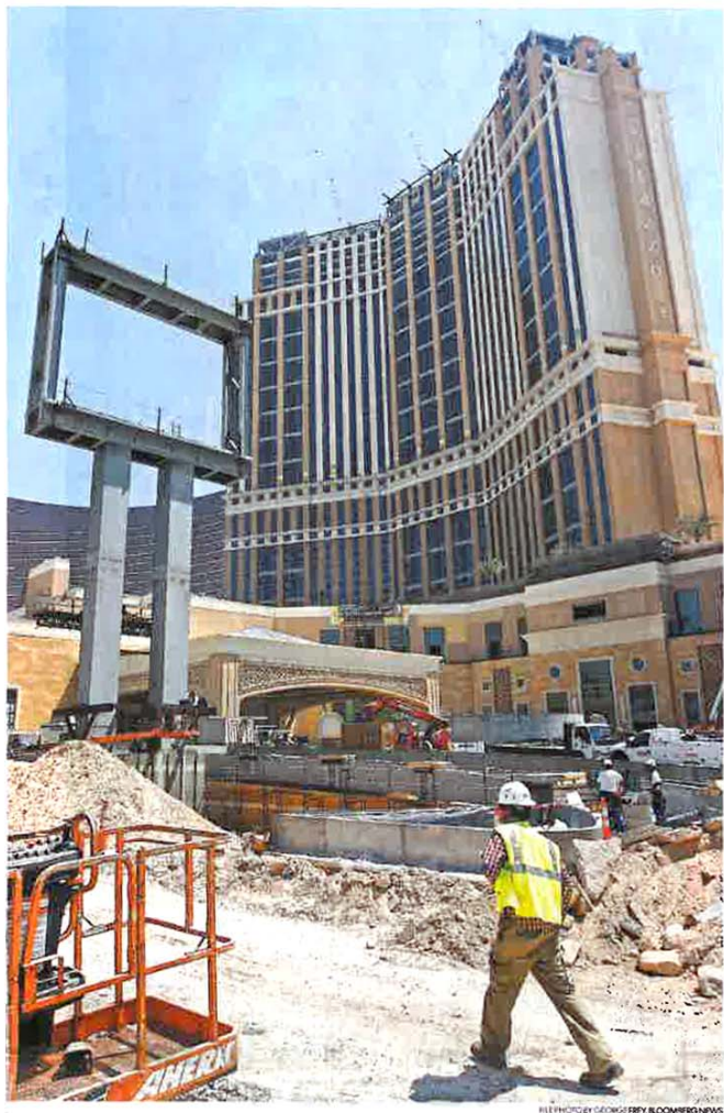
Las Vegas' Palazzo Hotel, being built in August 2007, stood as the world's largest green building for a time.
